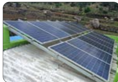
Solar Panel system supported to flour mill
